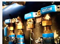
RELIEF VALVE LOCATED UNDER AER-FLOW MANIFOLD
