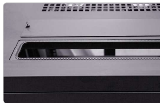
Nylon bush lining in all cable entry glands to protect from wear and tear
