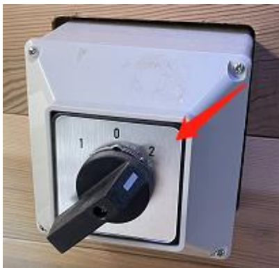
Power to Infrared heaters
