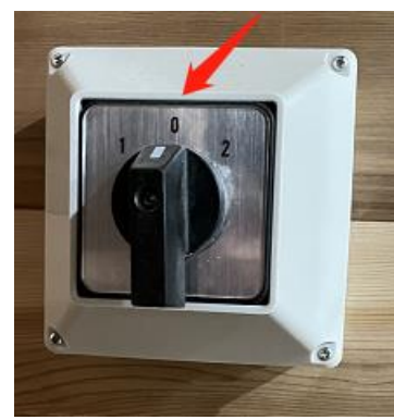
Power turned OFF
