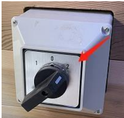
Power to Infrared heaters
