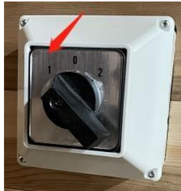
Power to stove heater
