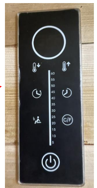
Sauna Control Panel has no Illumination
