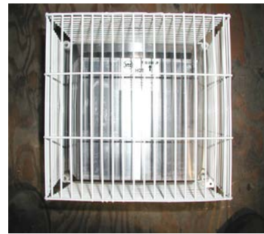
VIEW OF SAFETY CAGE
