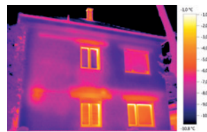
Thermal image with ScaleAssist
