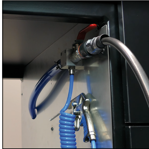
6. Open wastewater valve.
