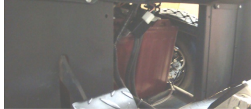
Front access panel opens to two more batteries
