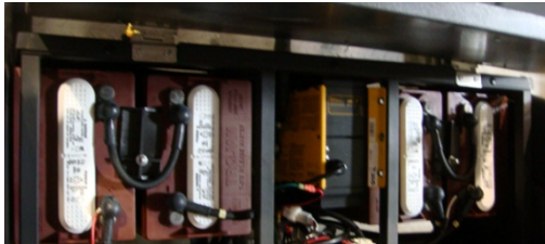
Four Batteries Under the Seat
