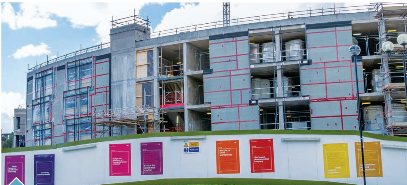
Aston University: 10mm Cemboard is used as the primary sheathing board, total quantity used 6,000m 2 .
