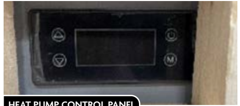
HEAT PUMP CONTROL PANEL
