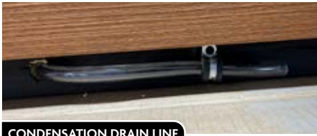
CONDENSATION DRAIN LINE
