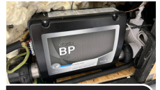
SPA CONTROL SYSTEM
