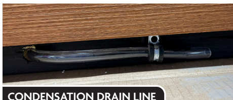
CONDENSATION DRAIN LINE
