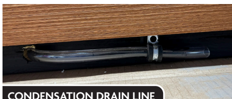
CONDENSATION DRAIN LINE
