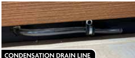
CONDENSATION DRAIN LINE
