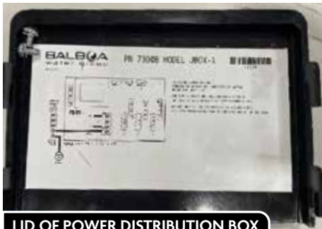
LID OF POWER DISTRIBUTION BOX
