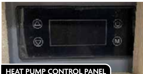
HEAT PUMP CONTROL PANEL
