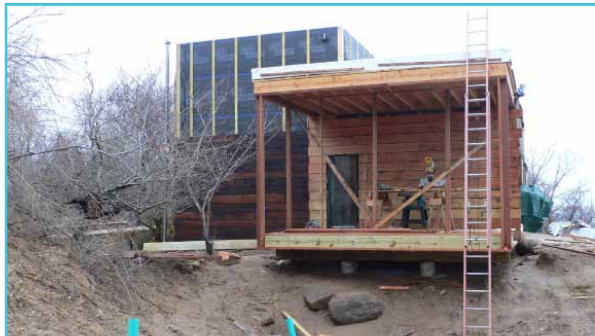
SOLITEX Mento 1000 at Ryall Porter Sheridan's passive house project in Orient Point NY
