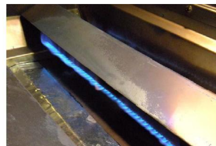
Normal Burner Flames
