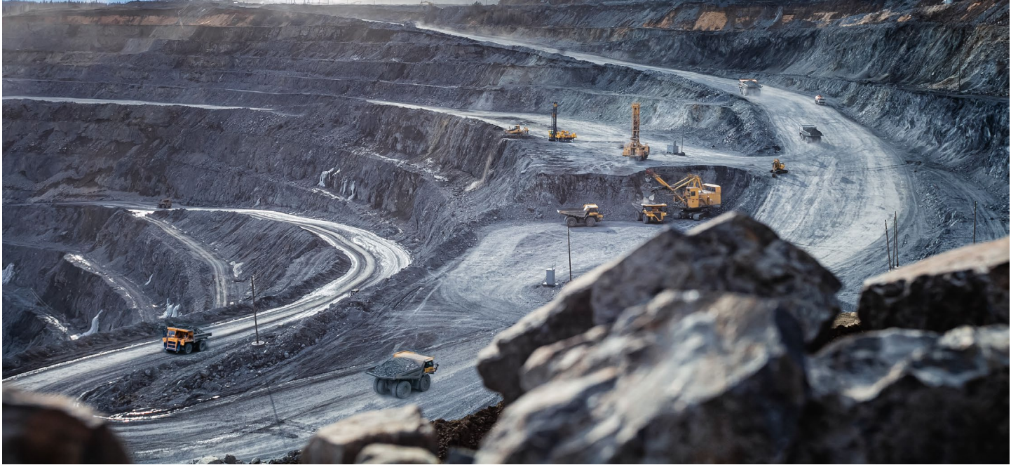
The large-scale and costly excavation of kimberlite rock to find embedded rough diamonds.
