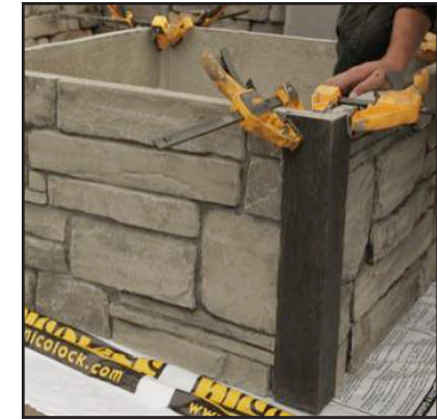
Use clamps to hold each side of the corner to the side panels.
