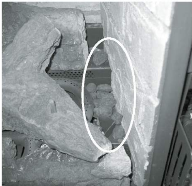
Right side of Burner
