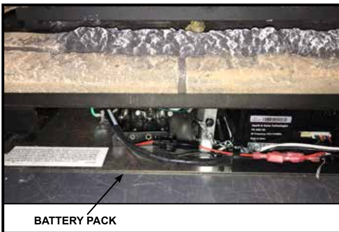
Figure 6.3 Battery Pack Installed
