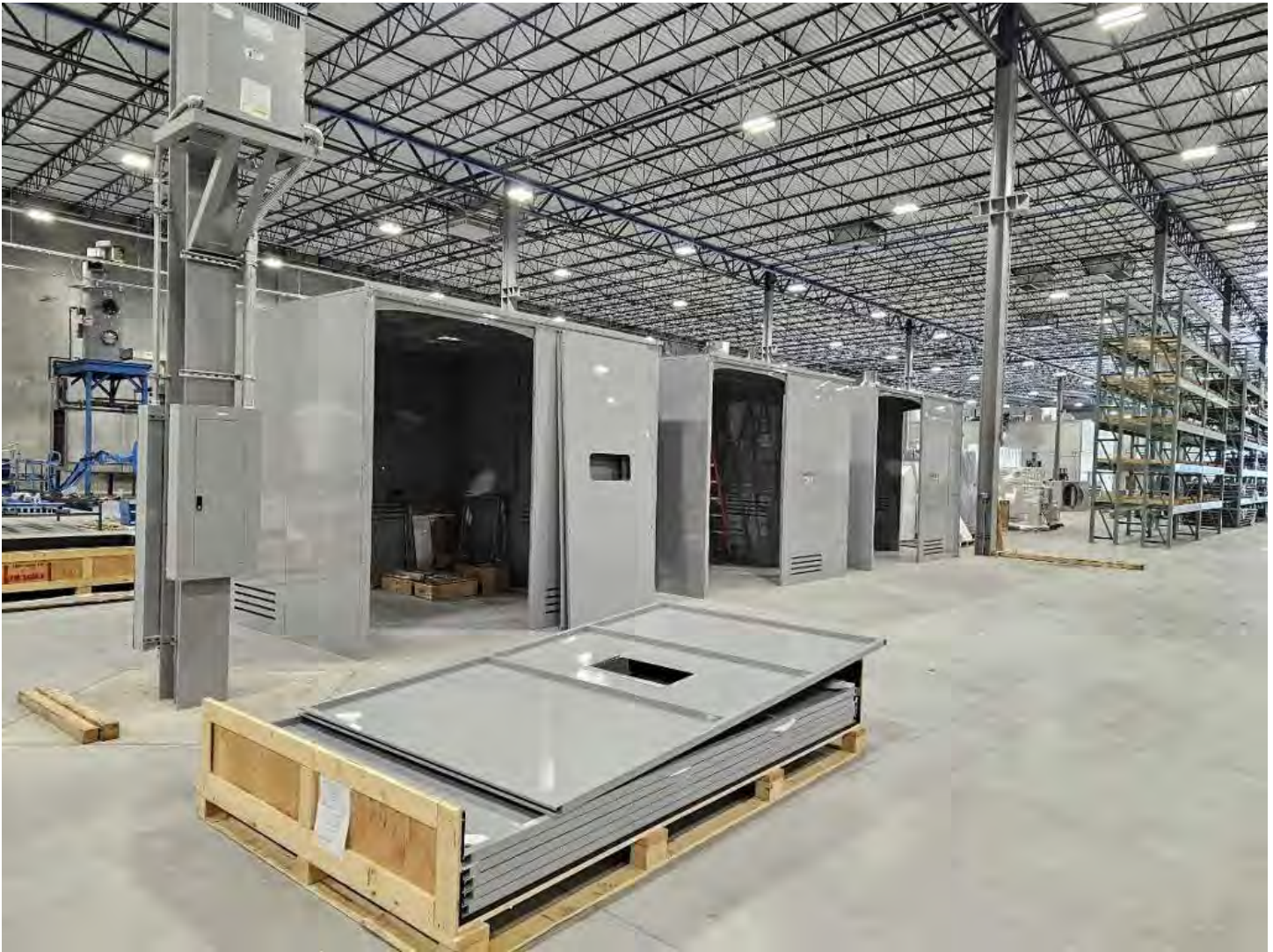
United Alloy – This is a custom system with 3 doors and ceiling in each work cell.
