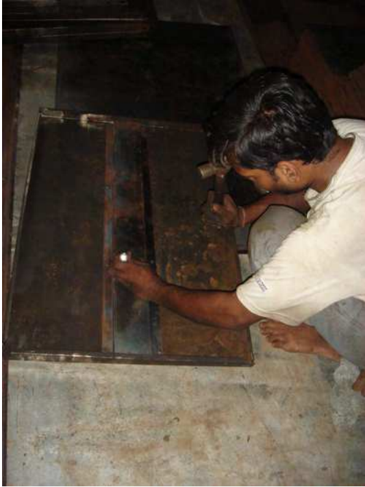
Another metal sheet is riveted to the larger metal sheets for support so that the rack can carry more weight.
