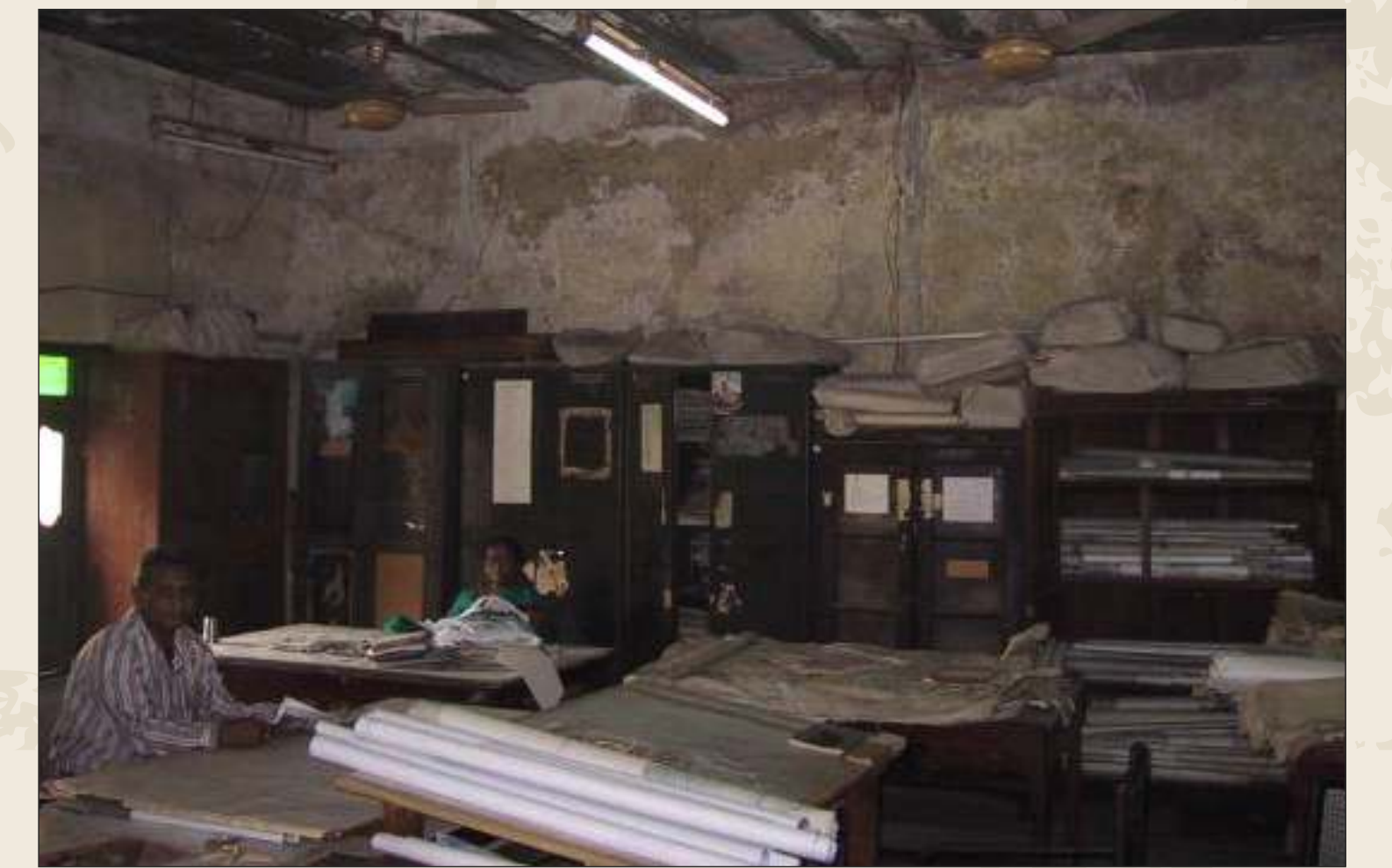
Dilapidated & run down state of tenanted spaces post 1960.
