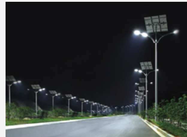
80W LED solar street lighting project – Melaka Malaysia 2010
