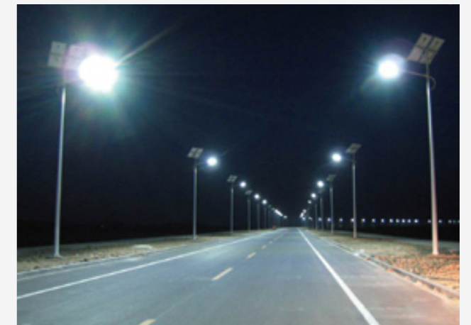
90W LED solar street light project – Denizli Turkey 2012
