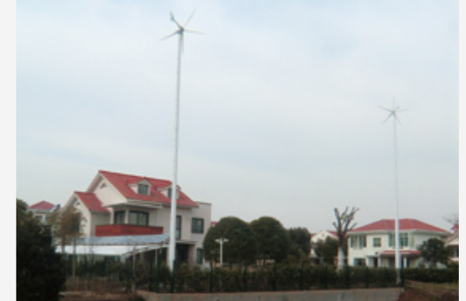
10KW wind solar hybrid off-grid power system for villa – Shanghai 2009
