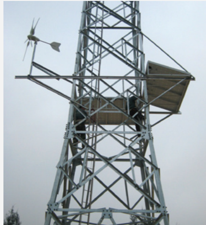
3KW wind solar hybrid off-grid power system installed on existing telecom tower as a backup power system – Hainan China 2012
