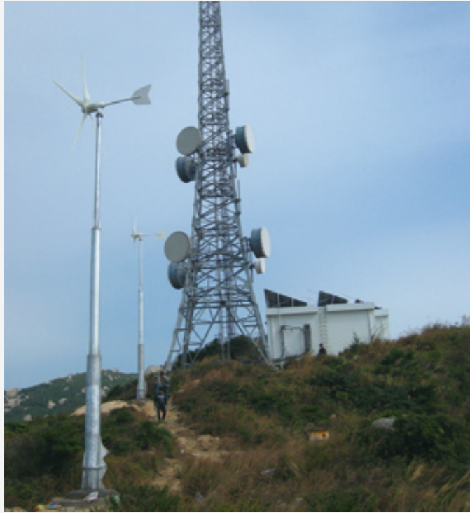
10KW wind solar hybrid off-grid power system for telecom tower – Baili Island, Zhuhai 2011
