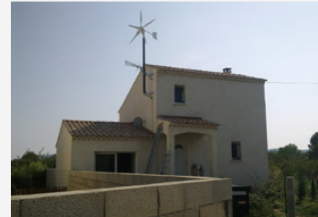
HY-1000 grid-tie system with wall fixation installation - Lyon France - 2011
