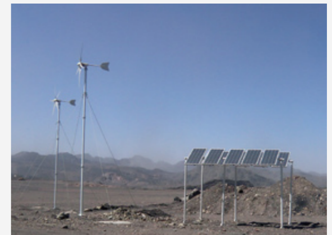
3KW wind solar hybrid off-grid power system for mining field – Chile 2008
