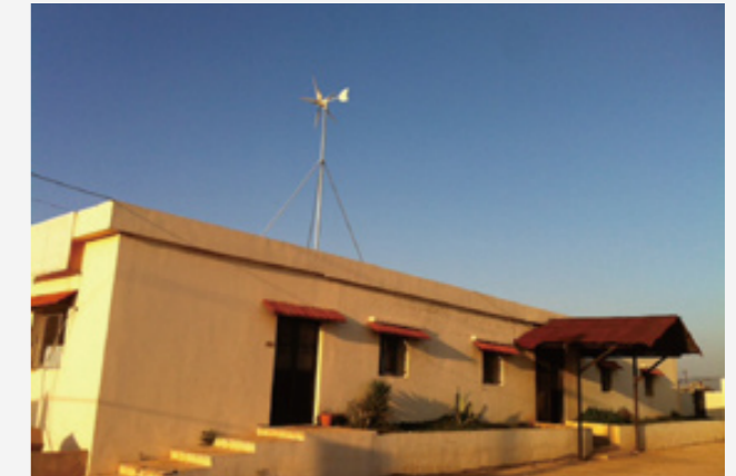
HY-1000 grid-tie system with flat rooftop installation - Lebanon - 2008
