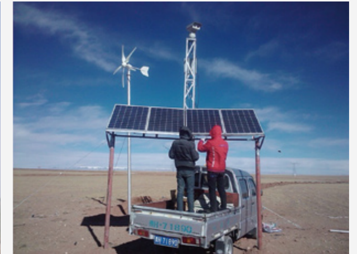
Wind solar hybrid off-grid monitoring system for oil field – Qinghai 2011
