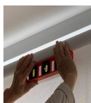
Using spirit level to check if the blinds is on the same level
