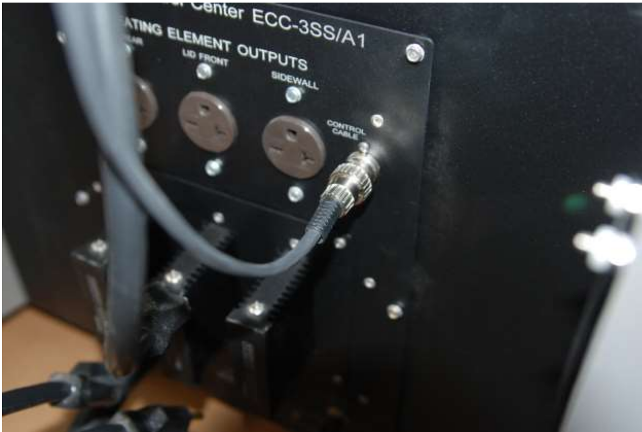
Figure 13 - Control Cable Connection
