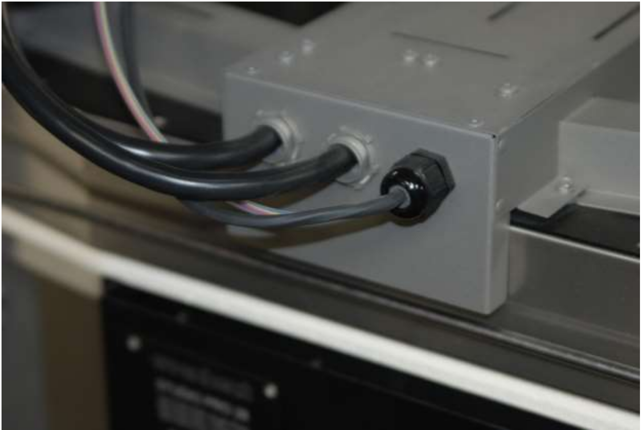
Figure 50 - Cables Run Over Top of Lid Hinge Rod
