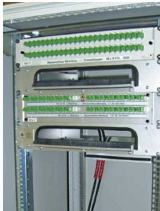
Example of a cable termination — in this case as a plug-in module in an existing connecting box
