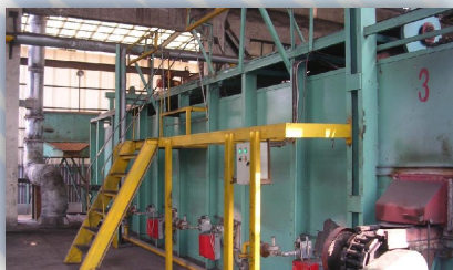
Heat Treat Furnace
