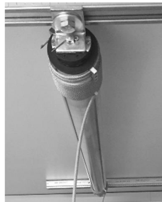
Even without tension the cable wraps are neatly side by side and no overlapping.
