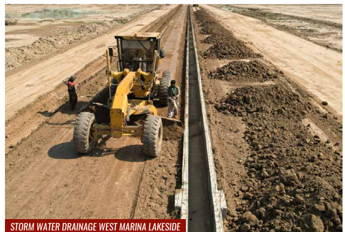
STORM WATER DRAINAGE WEST MARINA LAKESIDE
