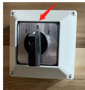
Power turned OFF
