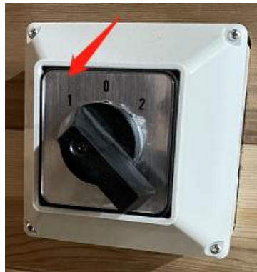
Power to stove heater
