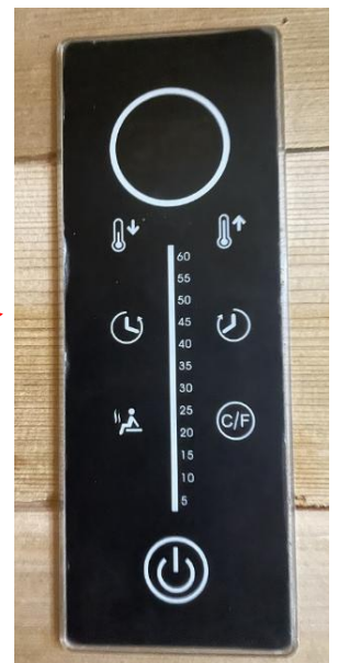
Sauna Control Panel has no Illumination
