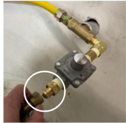
Gas Supply Line to the RV47 Regulator Note: Installer to supply gas line
