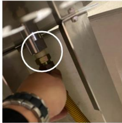
Yellow Flex Line (Other End) to Burner Manifold
