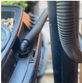
Top feed from downpipe waters all planters.
