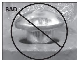
OVAL NECK OF BOLT NOT SEATED PROPERLY
