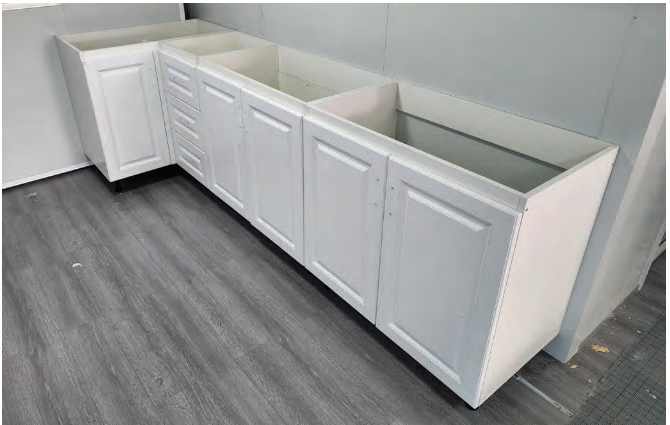
Floor cabinets for 40ft VIOLET unit, butted up against one another
