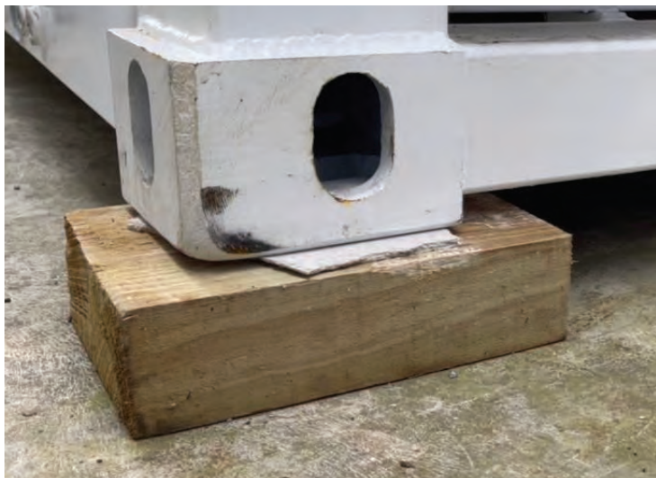
Shim pieces between footings & unit
