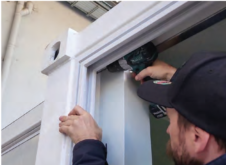
Pilot hole, top of doorway side
