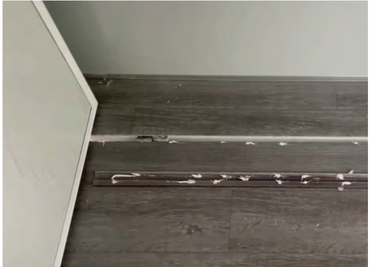
Adhesive on floor trim and floor gap
