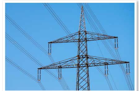
Redirect energy to the grid
