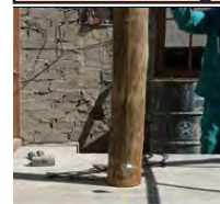
FIGURE 9. All king posts are to have plum bobs attached at the top during the entire construction period. This eliminates distorted roofs. Uprights should not be more than 3,500 metres away and the total ring beam width should not be less than 150 mm Ø in every structure. When the building grows in diameter, the thickness of the ring beam must expand (when authorised by the engineer). Poles for use as rafters shall have a diameter of at least 100mm measured at the thin end of the pole.
