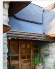
Figure 30. A steel box gutter can be made to fit this problem area over a front door and concealed by using poles and laths.
