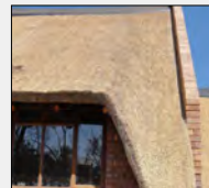
Figure 29. Bird mesh fitted around 'voetlaag' stitch around first batten with thin galvanized wire.
