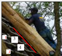
Figure 26. Displaying thatch wraps around laths when thatching. Pack length for at least three gaps, i.e. the tip must reach at least four laths.
