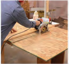
1. Cutting & Marking Plates Cut plates of plywood to required size. Plates are then marked as per desired use and layout. Plywood is used in roofing, flooring and wall plates.
