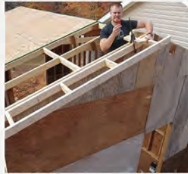
2. Installing Structure The support structure installed can be wall studs, timber floor joists or roof shingles. These support elements are cut, lifted to position and fixed by toenailing.
