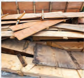
1. Disassemble & Collection Walls are disassembled and stacked. Nails are not removed as mills or mulch sites usually run timber waste through magnets to remove metals prior to processing.
