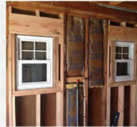
3. Framing Openings In walls, it is required to locate openings in the layout, which are then fitted with required trimmer studs and cripple studs to frame openings prior to fixing plywood.
