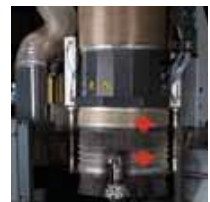
Controlled extraction hood
