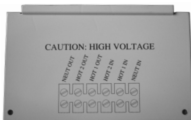
Figure 16 MS Series Inverter / Charger - AC Wiring Diagram (located on back of cover plate)
