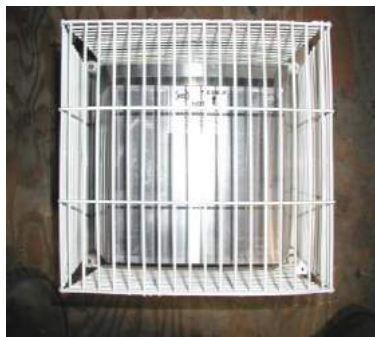
VIEW OF SAFETY CAGE
