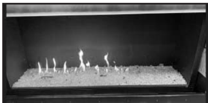
Figure 11.8 Incomplete Burner Lighting
