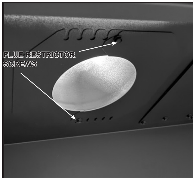
Figure 4.17 Flue Restrictor Installed
