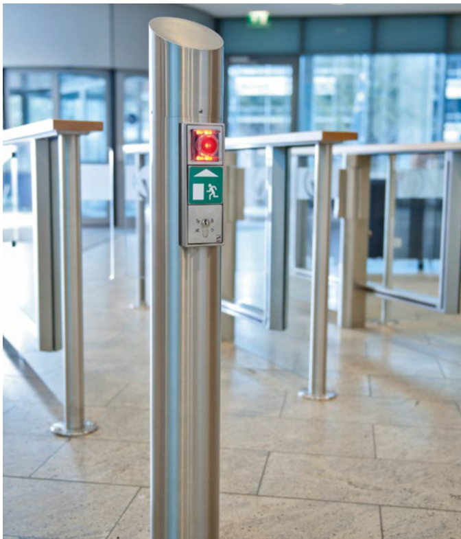
Card reader post with escaperoute terminal
