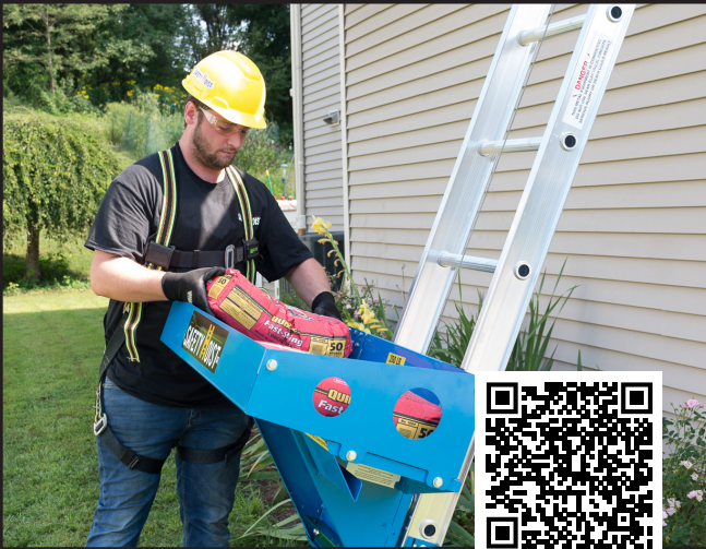
Gas Material Hoists
