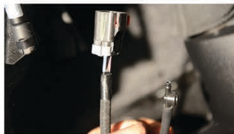
LOCATE WIRING HARNESS
