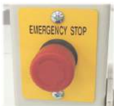
Below operation panel
