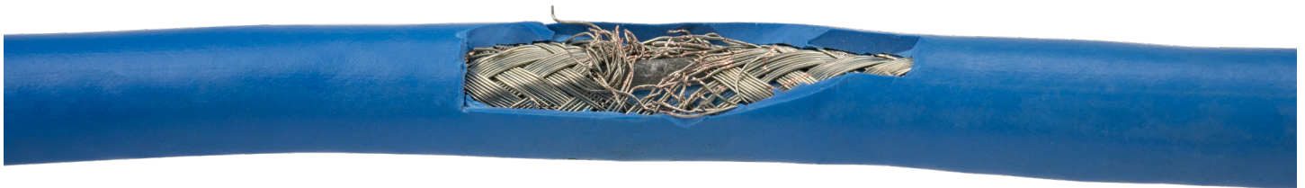
Photo 1: Cable jacket and shield braid damage
