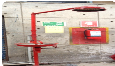
Eye Wash Station
