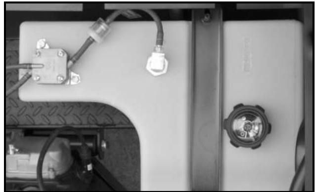
Figure 16b Fuel Tank
